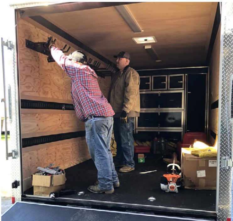
Members of the Humboldt County PBA designed and installed tool racks on the inside wall of the burn trailer.
